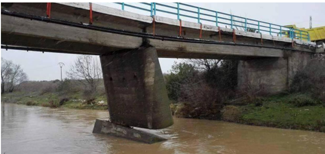
Figure 1.1 Yayakent Bridge view after flood in January 2016 [2].
