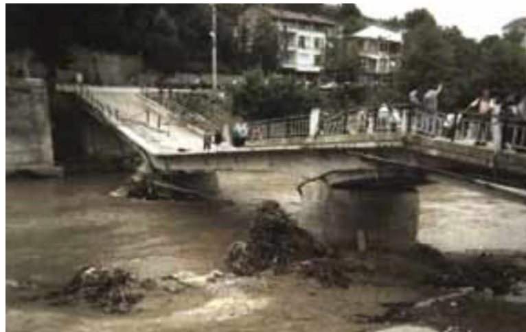
Figure 1.3 Failure due to scour at Devrek Bridge [4].
