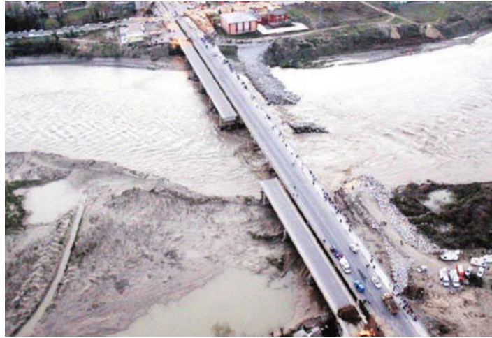
Figure 1.2 Çaycuma Bridge after the flood in 2012 [5].
