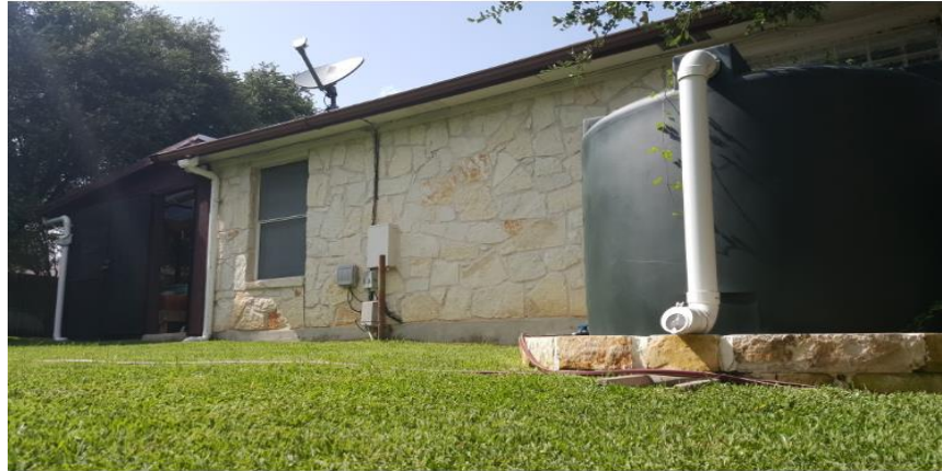
Figure 2.12 Residential rainwater collection system uses tanks, Arizona, USA
