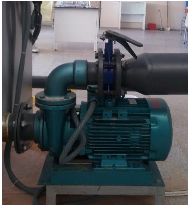
Figure 3.6 : Pump motor and butterfly valve
