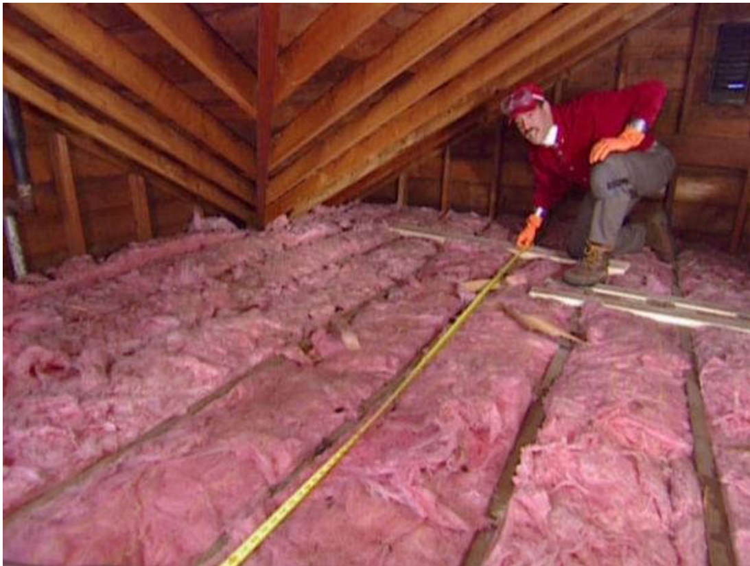
Figure 3.4 : Roof loft insulated with fiberglass.
