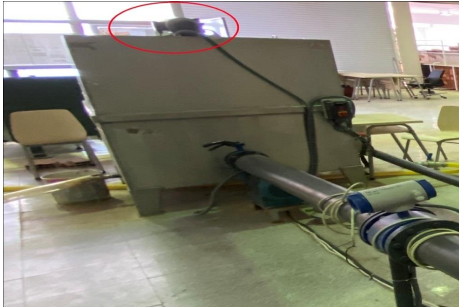
Figure 3.3 Storage tank and mixer
