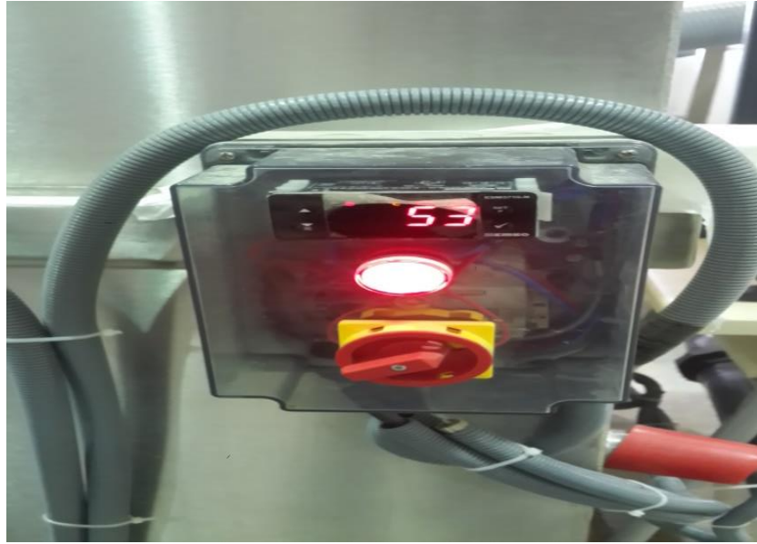
Figure 3.5 Temperature control panel
